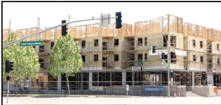
West Gateway Place Affordable Housing Project under construction at the corner of Tower Bridge Gateway and Grand Street
